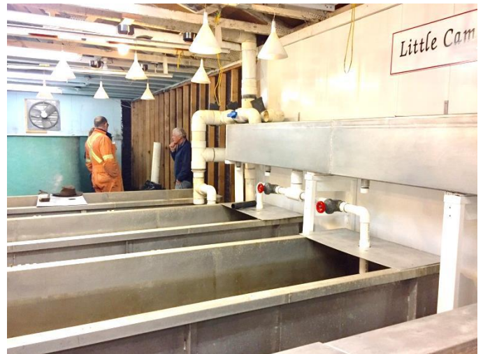
Lloyd McKay and Ron Meadley inspecting the west side in preparation for the installation of the new panelling, supports and new head trough
